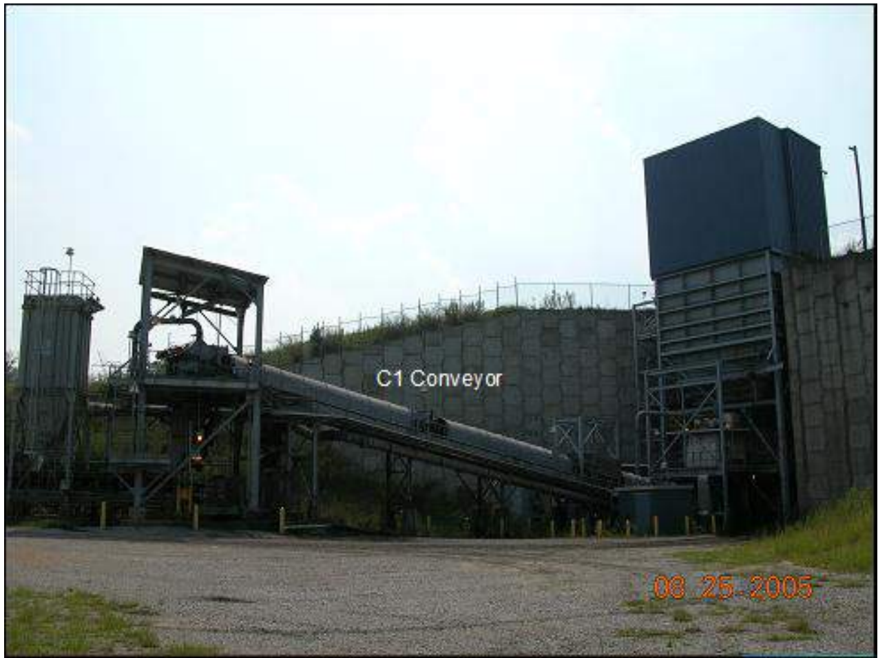
Figure 4. Primary Crusher and Feeder – C1 Conveyor
