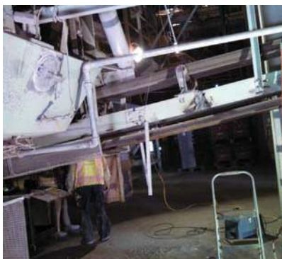
Figure 7 (right): the in-situ Sabia LiNX Analyser installed with a minimum of structural modifications
