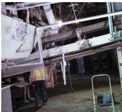
Figure 7 (right): the in-situ Sabia LiNX Analyser installed with a minimum of structural modifications
