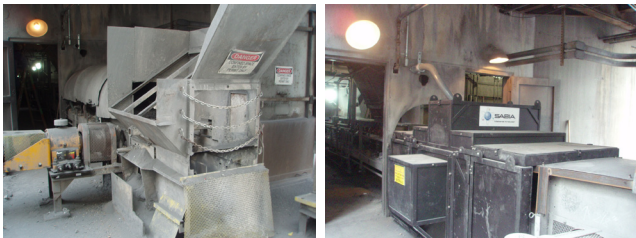
Lafarge Whitehall analyzer location before and after installation
